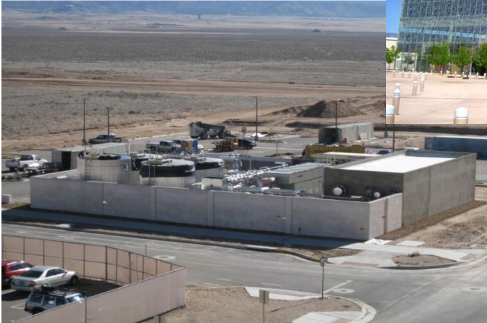
Micro Grid Plant
