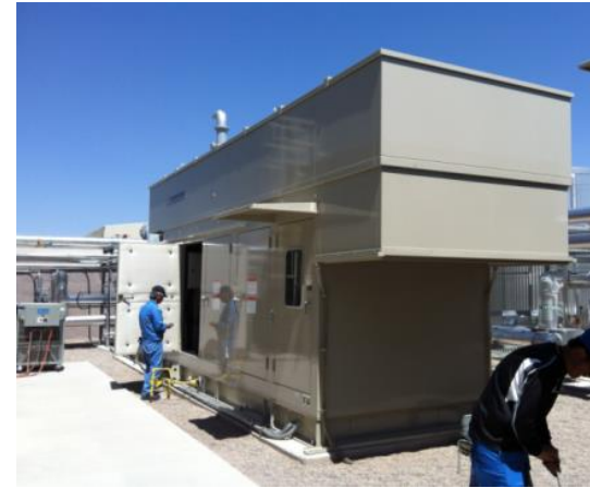
Gas engine generator
