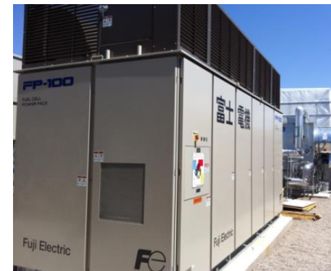
Hydrogen Fuel Cell
